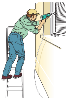
Figure 2a Incorrect - steps side-on to work activity
