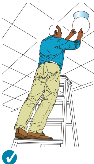
Figure 12 Correct - three clear steps. Don't work any higher up this type of stepladder
